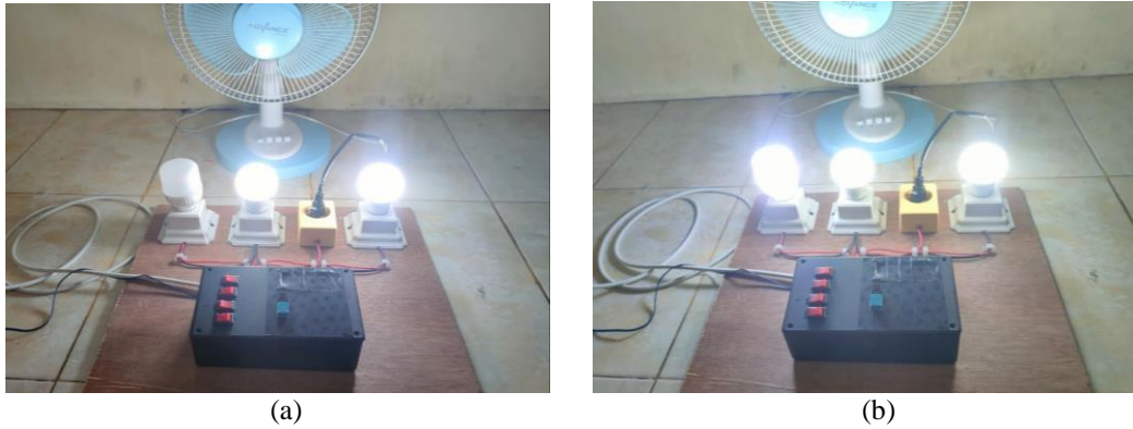
Figure 6. Smart room circuit with manual switches. a) switches v2 and v4 On, b) all switches in the On condition.
