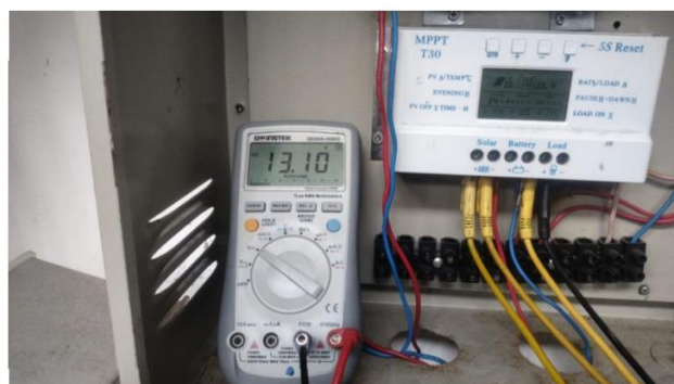
Figure 4. Checking DC voltage input
